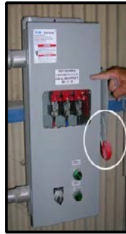
Disconnect Panels with “Lockout Here” Label and Energy Isolation Information
