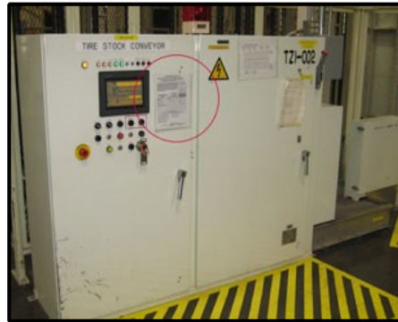
Equipment-Specific Energy Isolation Procedure shown in file on front of the Equipment Control Panel
