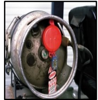
Locked Gas Cylinder
