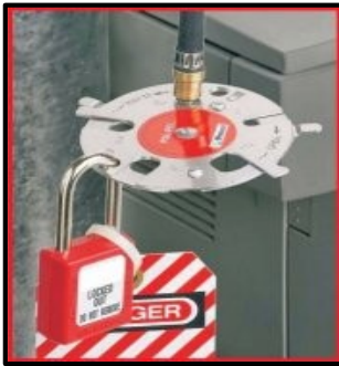
Locked Comp. Air Line
